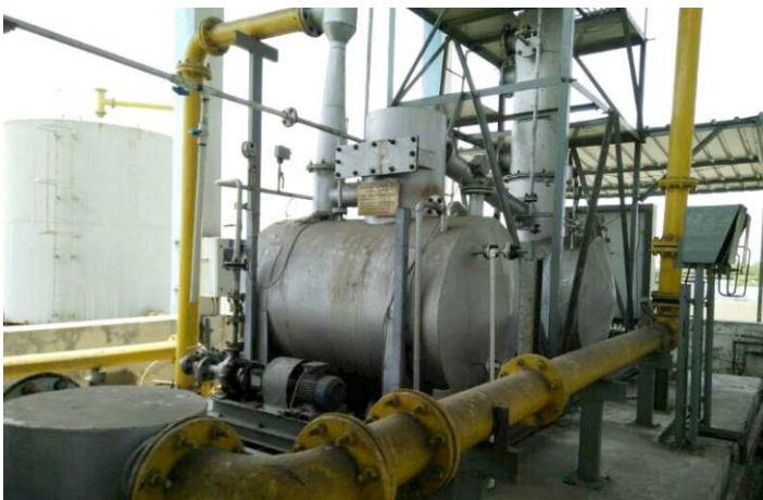
Ultra filtration unit
